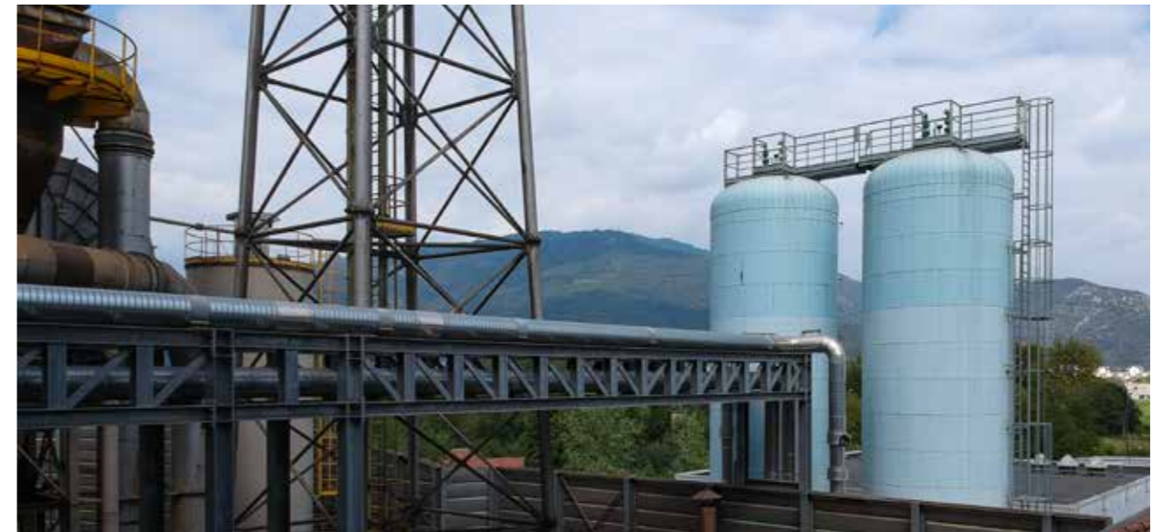
Alfa Acciai: array of pipes supplying the heat recovery plant from the steel mill and storage tanks
