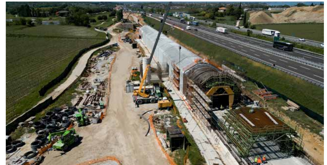
Ferroberica's construction yard - The artificial tunnel for the Brescia-Verona High-Speed train line in Peschiera del Garda (VR)
